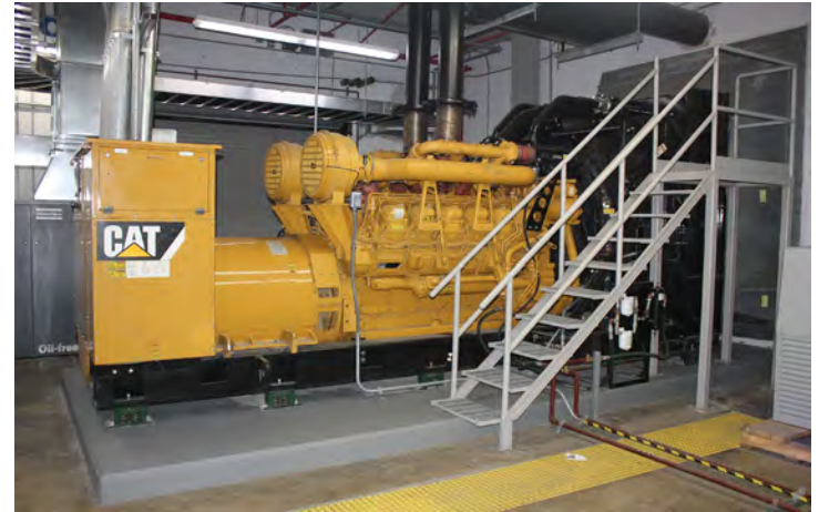
Emergency Back-Up Generator
